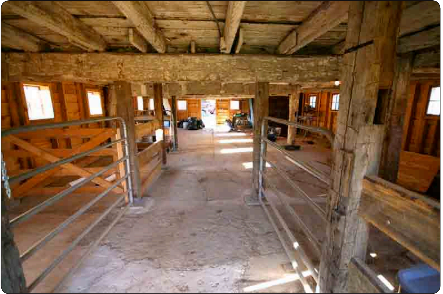
WOGAN AND HIS CREW BROUGHT THE BARN INTO COMPLIANCE WITH EXISTING BUILDING CODES.
